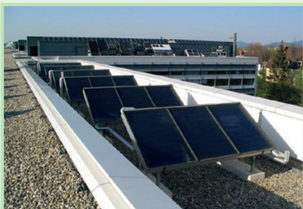
Solar hot water panels just 20 m 2 in size are sufficient to provide energy for the cooling process
