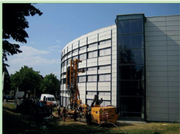
80 metre deep holes were drilled into the ground to accommodate the geothermal probes
