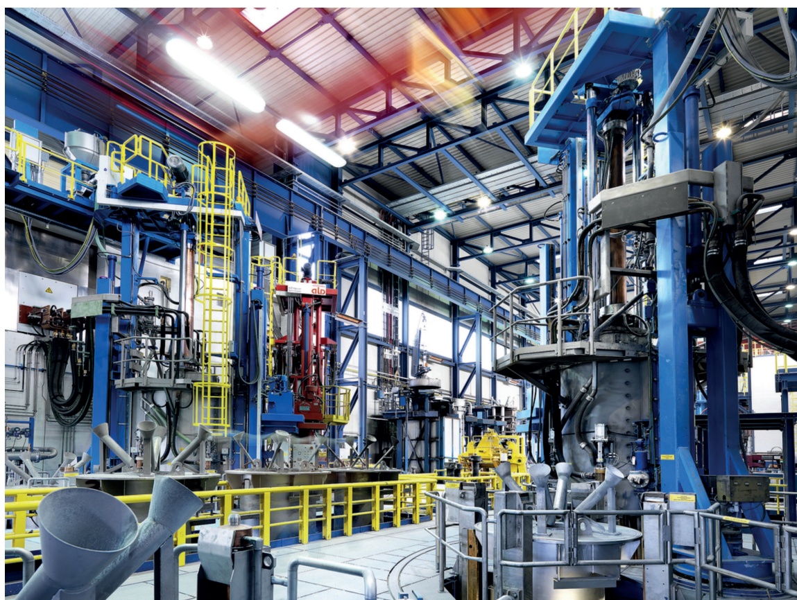
The plant in Unna is equipped with various ESR (blue) and VAR (red) units
